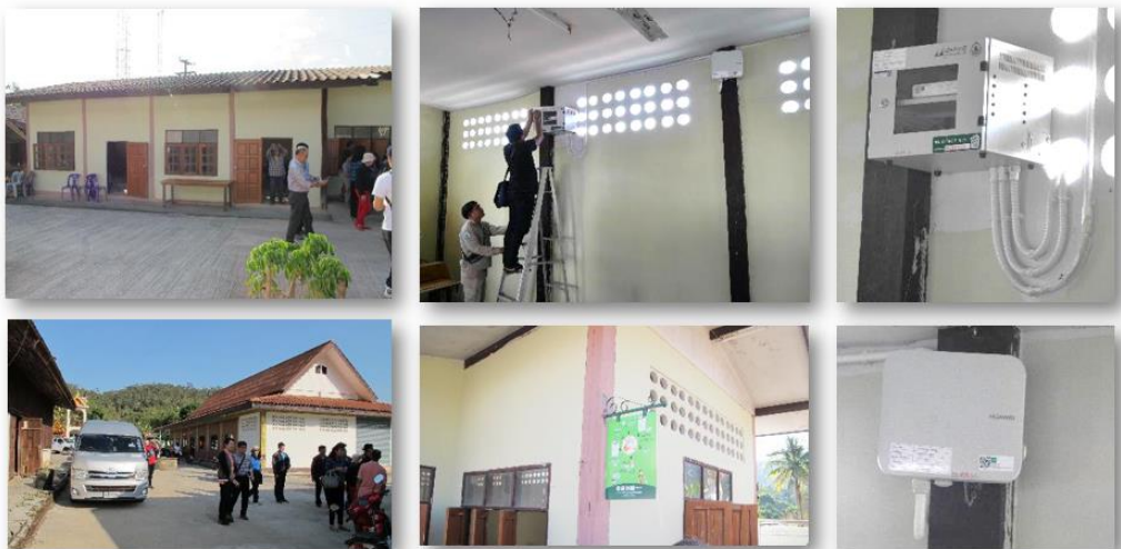
Figure 22. A village hall with installed Wi-Fi hotspot equipment and Net Pracharat signage
